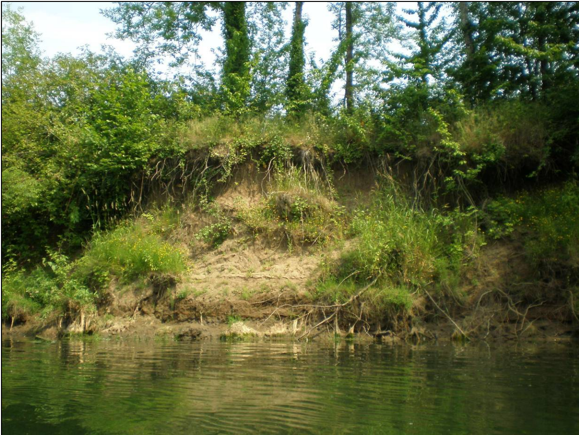
Figure 2. View of existing bank failure at WTP on the Calapooia River, river-right streambank.
