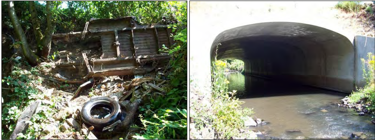
Figure 4-24. Debris such as old car bodies was used in the past for bank stabilization treatments (left). A concrete arch at SE 2 nd Avenue provides fish passage (right).
