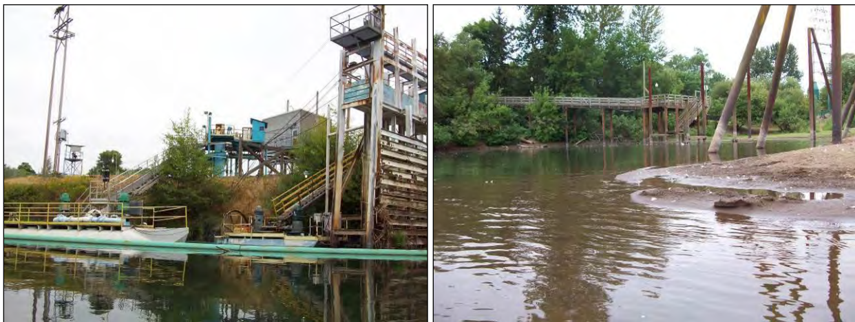
Figure 4-17. The pump station on the Willamette River supplies water to the ATI-Wah Chang facility (left). Pilings protect the City of Albany pier on the Willamette River downstream from the Calapooia River confluence.
