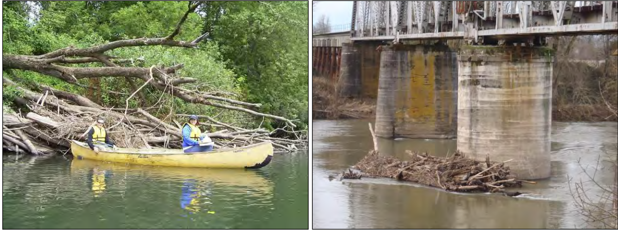
Figure 4-15. Large wood accumulations on the Willamette River provide channel margin complexity and habitat (left). Wood and debris transported by the Willamette River often accumulates on bridge abutments, such as this private railroad bridge, located in the assessment reach (right).
