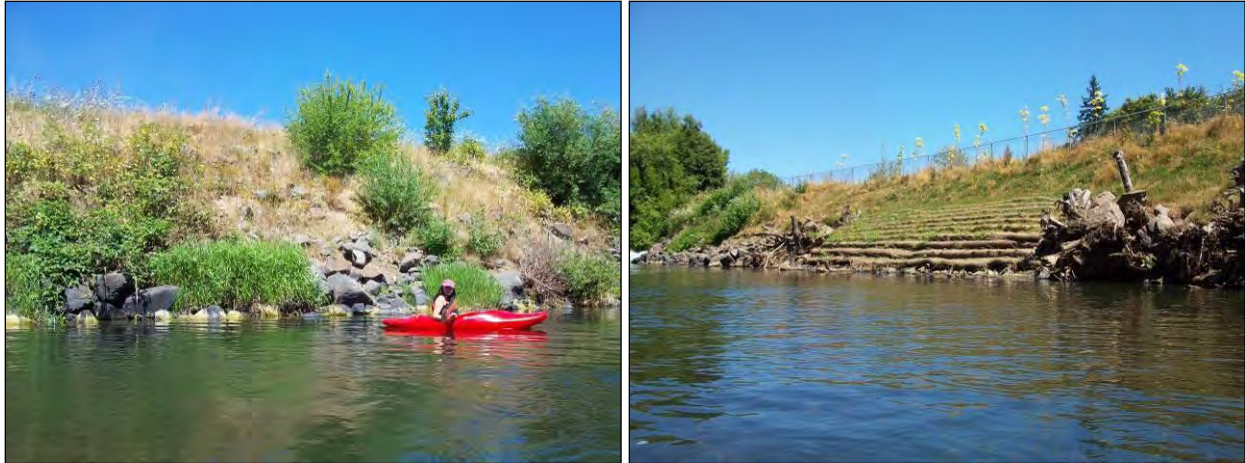
Figure 4-7. Two examples of bank stabilization treatments in the assessment reach. The left photo shows older rock riprap and a revegetating streambank at STA 85+00. Bioengineering and large wood structures were used to stabilize an eroding bank adjacent to City of Albany settling ponds at STA 32+00.
